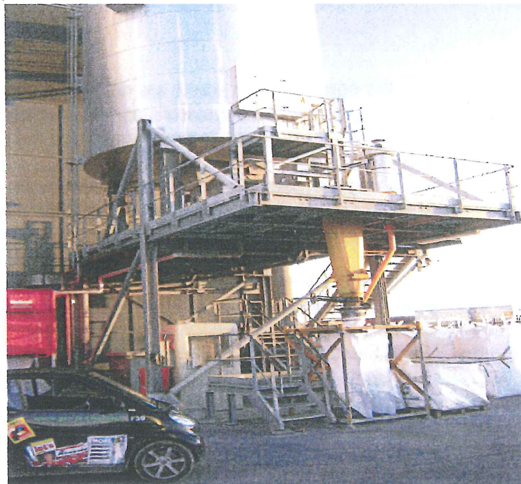
SILO FOR COLLECTING APCr IN BAGS
